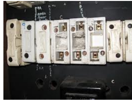
Electrical Equipment Arc Shields, ACM in fuses and electrical contacts
