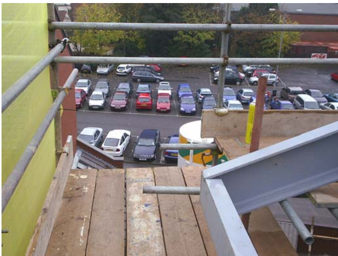
Work at Height
