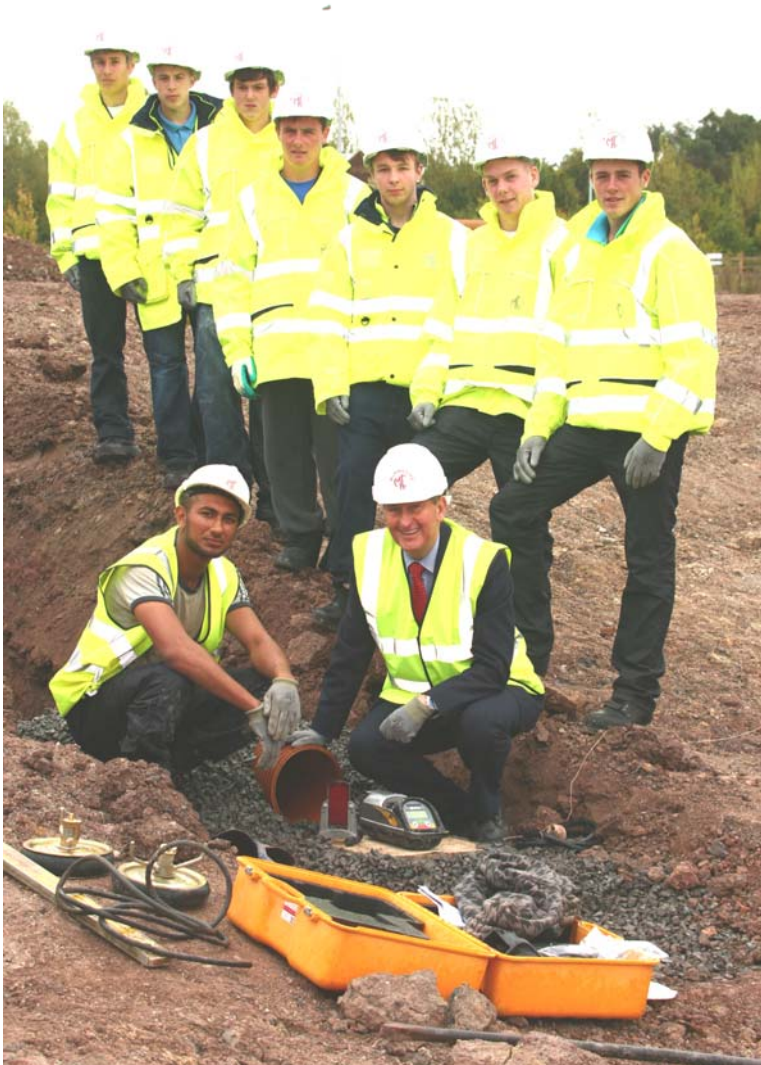
L to R Back: Apprentices Sam Moseley, Jack Harris, Jack Caton, Josh Ellis, Liam Chadwick, Owen Lloyd and Jack Farnell. Front: ex-Apprentice Ravi Kumar, now pipe-layer, and director, John Butler
