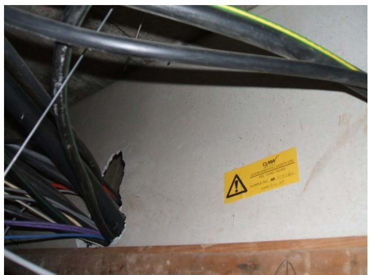
Damaged Fire Stopping spotted on a DMW Survey. This is dangerous from two standpoints, at least!
