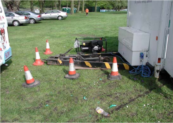
Un-earthed and un-guarded generator!
