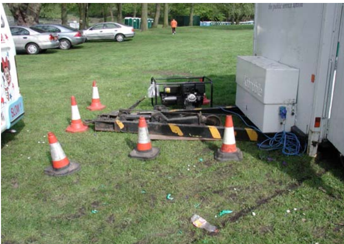
Un-earthed and un-guarded generator!
