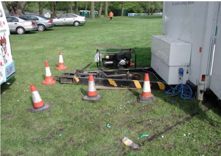
Un-earthed and un-guarded generator!
