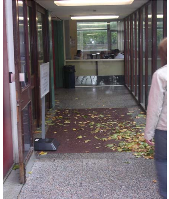
Original Baker Entrance Corridor – with Leaves and Water when it rains!
